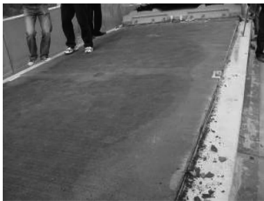
图 5 揭板后的 CA 砂浆表面 Fig. 5 Surface of the CAM after the slab was uncovered
